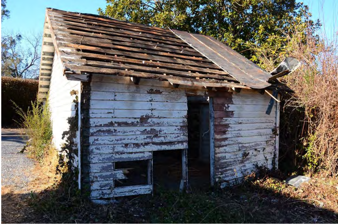
General wear and decay.
