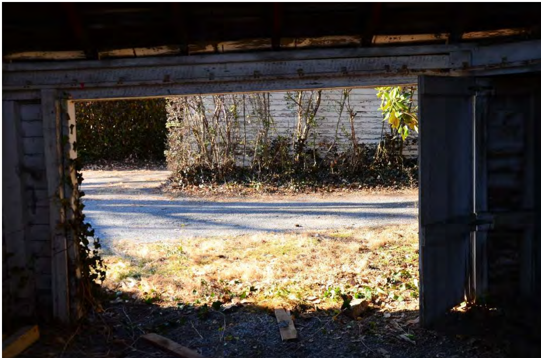
Building tipping. Low entry height.
