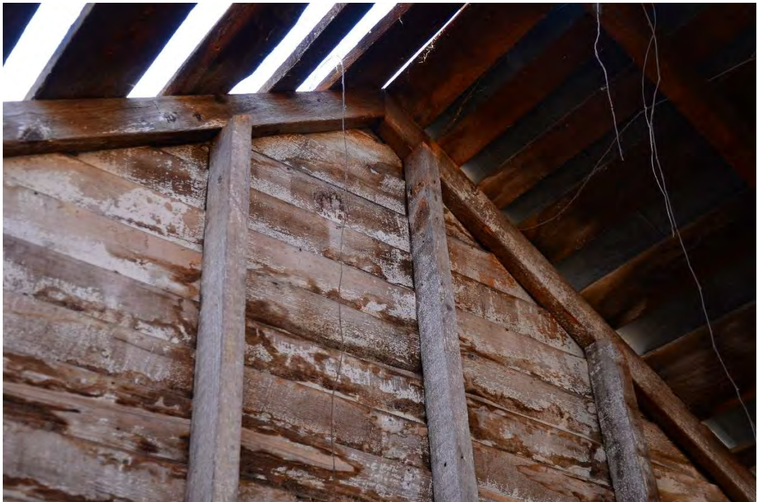
Evidence of water damage.
