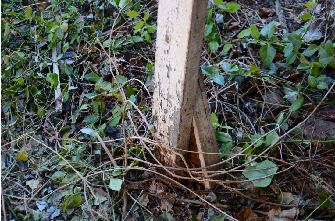
Wood posts supporting structure rotting at ground level.
