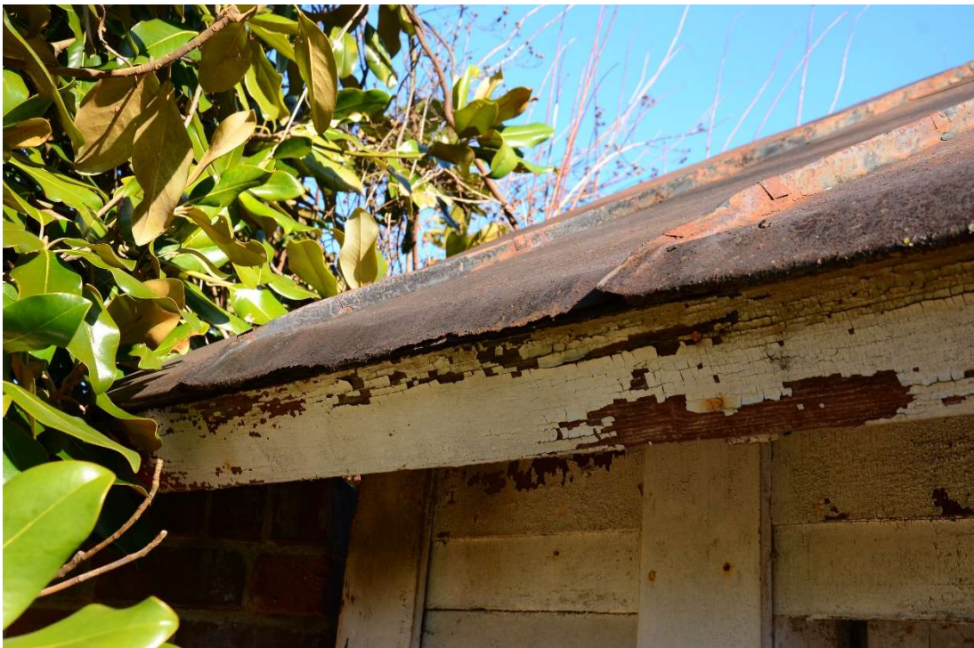
Rusting and decay at roof edge.
