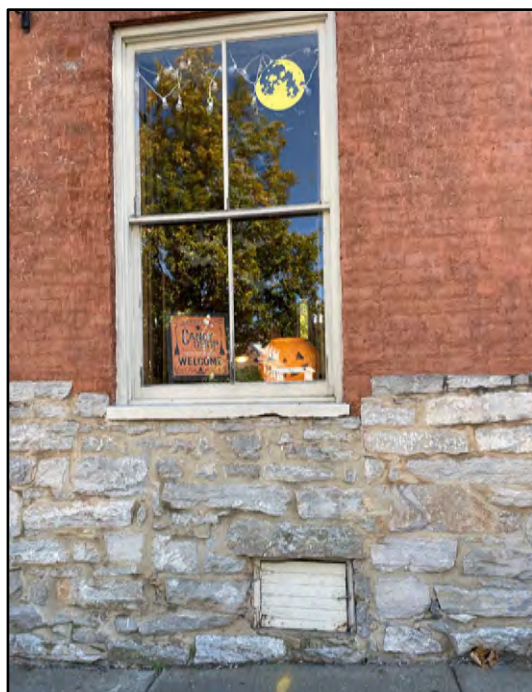
Existing “small door”
