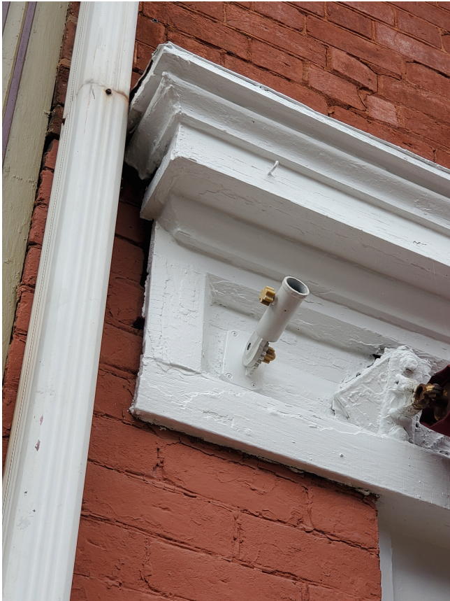
Storefront frieze and cornice on the Norgrove Building, above the Southern Inn (35 S Main Street) – model for modifications at 31 S Main Street
