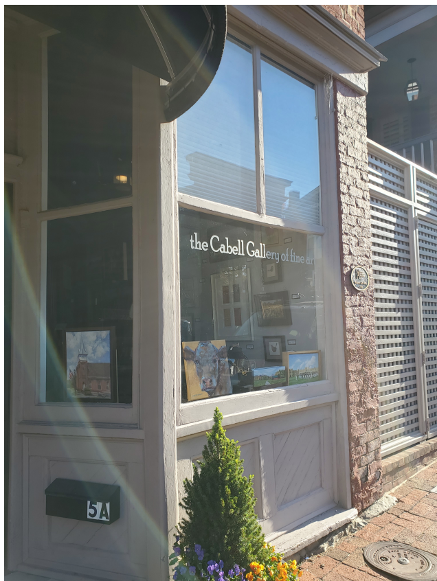
5 W Washington storefront – proposed design for 31 S Main Street would be similar, especially at the bulkhead level.
